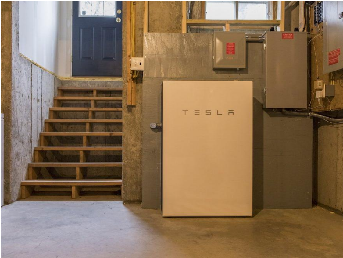
5 kW / 14 kWh installation: Tesla Powerwall 2 (5 kW / 14 kWh/unit); installed in utility space
