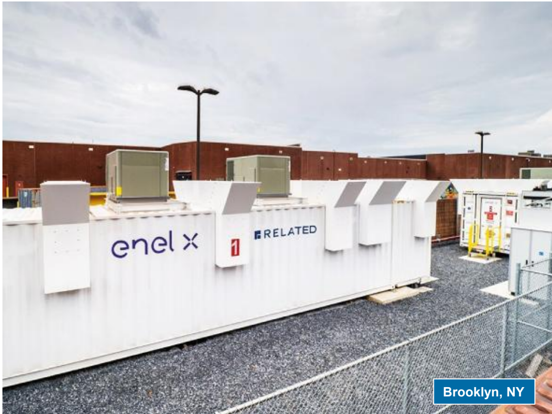
4.8 MW / 16.4 MWh installation: Enel X's Gateway Center project ; sited at a commercial shopping center in Brooklyn, NY
