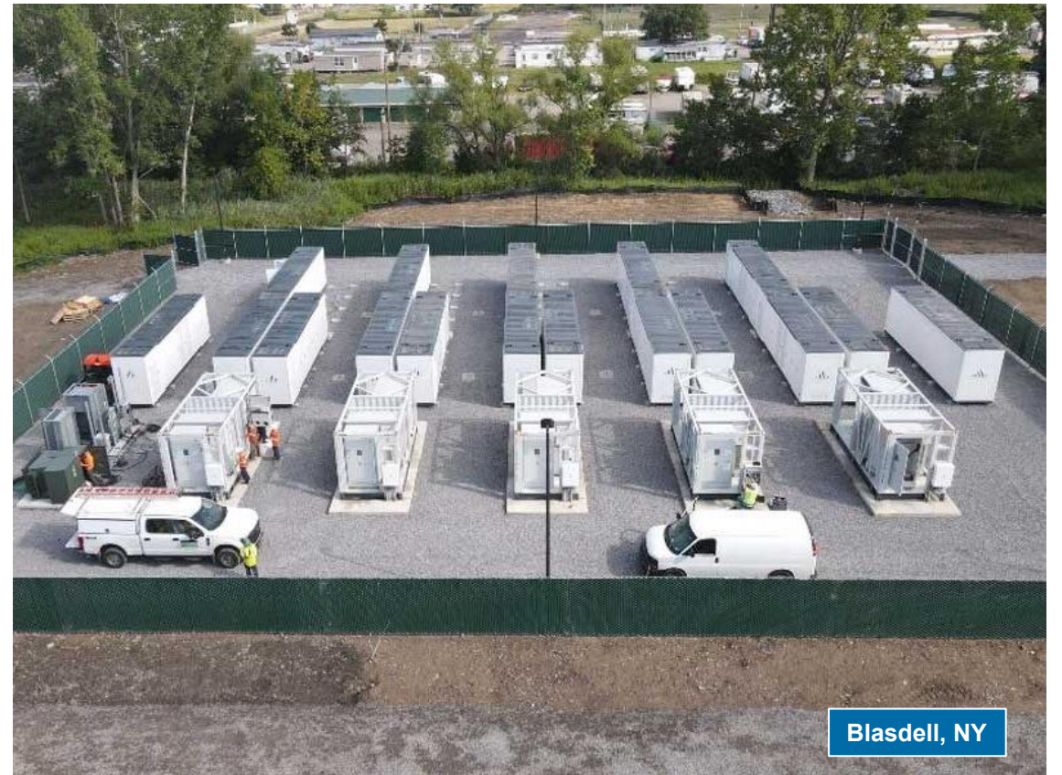
20 MW / 45.6 MWh installation: Key Capture Energy's KCE NY6 project ; Blasdell, NY, adjacent to self-storage facility, landscaping/topsoil supplier, and plant nursery.
